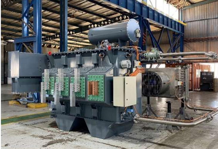
Impala Platinum Unit 1 factory test setup:
